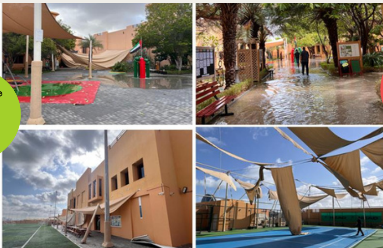
Storm damage at Gardens Campus
